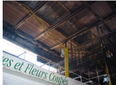
Figure CS10.2: The damaged interior of the warehouse, which was quickly repaired. (Courtesy CIMbéton, France)
